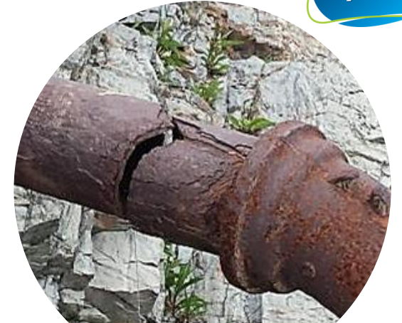
WORN OUT PIPELINES
